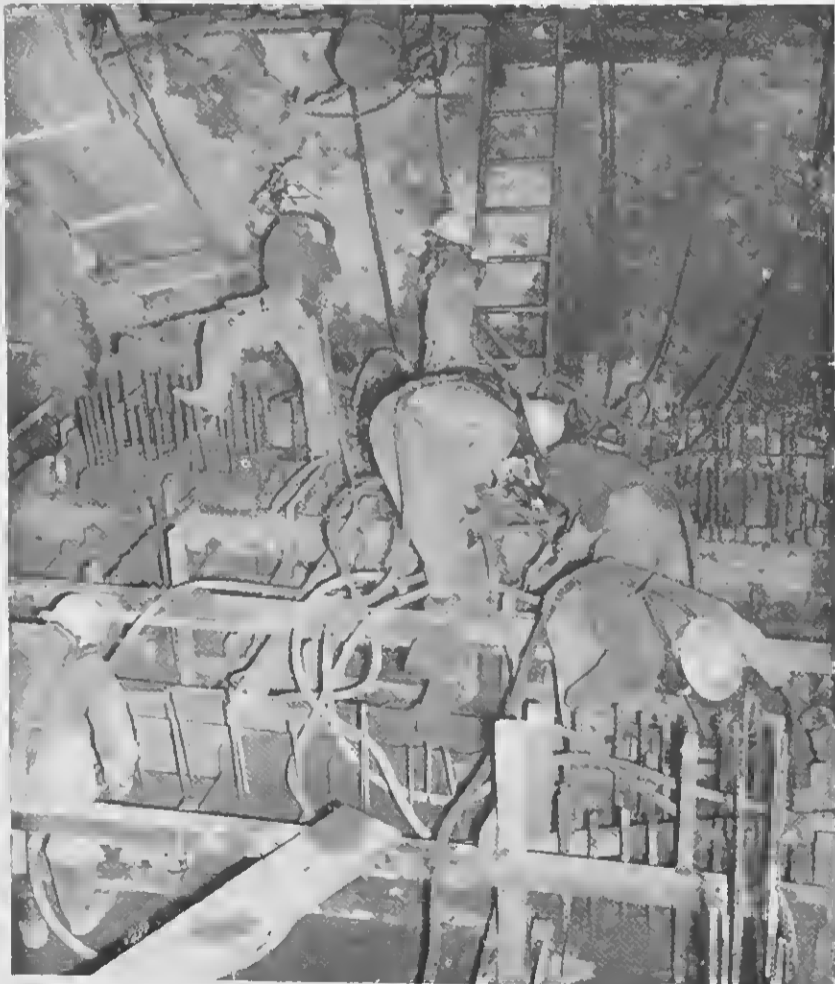
OUT OF THIS WORLD: Looking like men from out of this world, these members of the "concrete gang" of the Mechanical Department are busy putting in a new base for the No. 7 turbo-generator in the No. 1 Powerhouse. Working inches above sea-level, they're wearing fresh air masks to guard against hydrogen sulfide which seeps through the coral strong enough to discolor the coins in their pockets. The new General Electric turbo-generator will produce 7500 kilowatts; some 3500 more than the old No. 7 which "went bad" in January of 1952. The new unit is expected to go into operation early next year.
